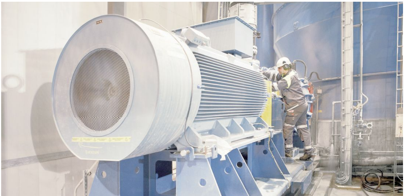
Object metering is used to show the electricity consumption where it occurs
