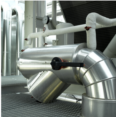
Air conditioning application
